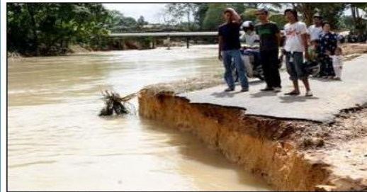
Kluang, Johor, Jan 15: The access road to Kampung Seri Cahaya has collapsed due to the continuous rain. NST pix by Amran Hamid.
